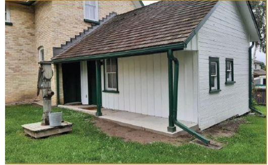
A view of the back porch after the restoration work on the south side was completed and the east side (with two windows) was scraped and repainted.
